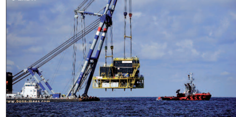
"MATADOR 3" installierte 2010 die Umspannplattform für den Offshore-Windpark Baltic 1. In 2010 floating crane "MATADOR 3" installed the substation at the offshore wind farm Baltic 1. © EnBW
